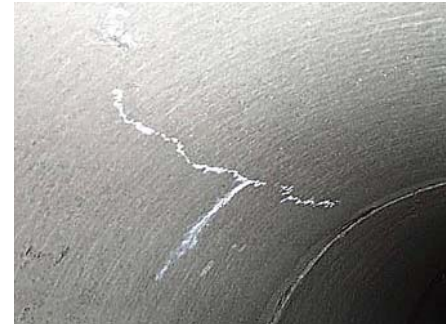
Autogenous healing in concrete pipe.
